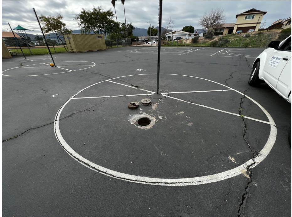
Photograph 7: View of West Hardcourt play area looking west. Note the several patched and unpatched AC cracks running in the north-south and east-west orientations.
