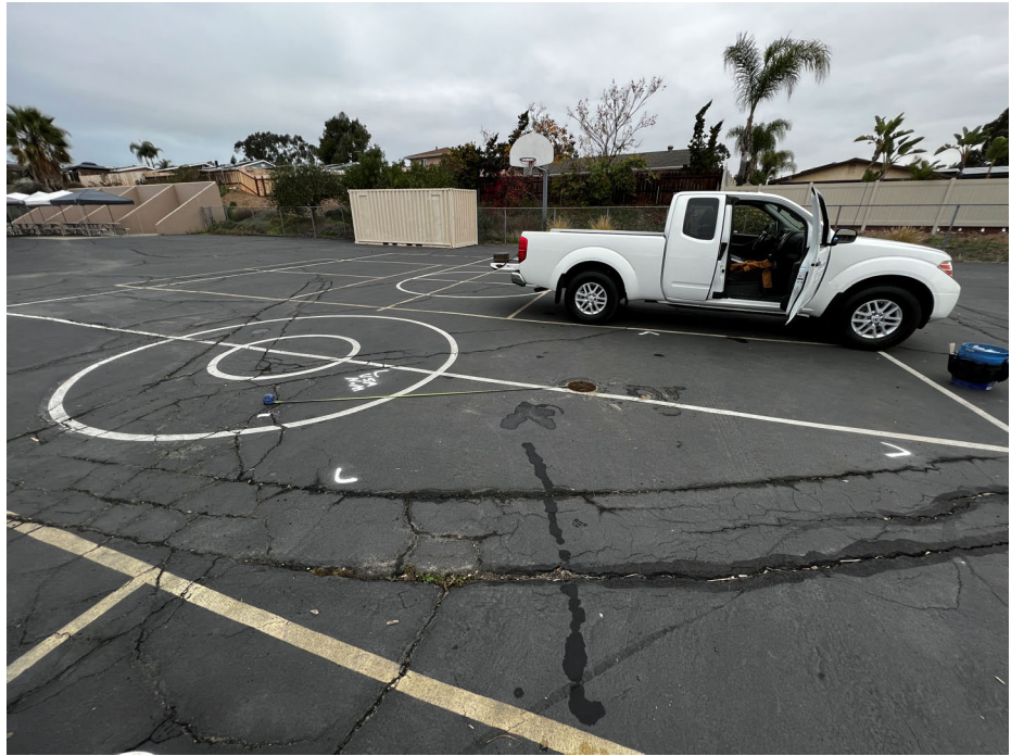
Photograph 1: View of East Hardcourt play area looking north. Note the several patched and unpatched AC cracks running in the north-south and east-west orientations.
