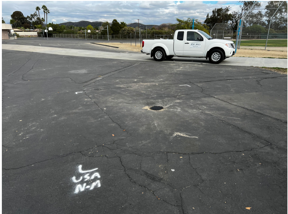
Photograph 6: View of South Hardcourt play area looking east. Note the several patched and unpatched AC cracks running in the north-south and east-west orientations.
