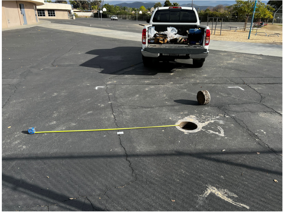
Photograph 5: View of South Hardcourt play area looking east. Note the several patched and unpatched AC cracks running in the north-south and east-west orientations.
