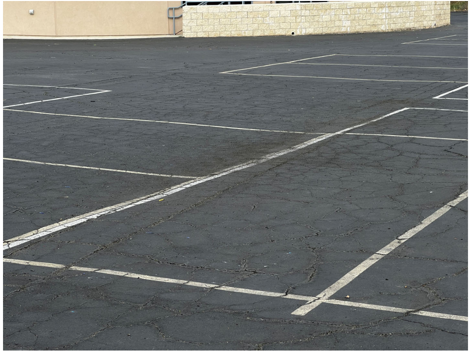
Photograph 3: View of several alligator cracks in the AC pavement for the East Hardcourt play area looking north.
