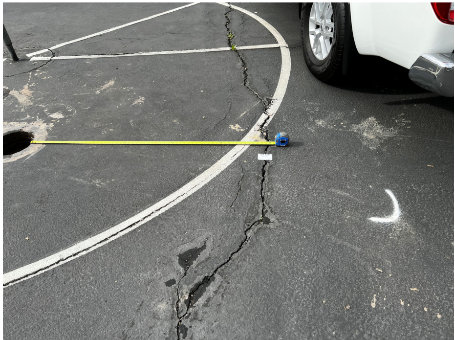
Photograph 8: Close-up view of an AC crack approximately 1/2-inch wide.
