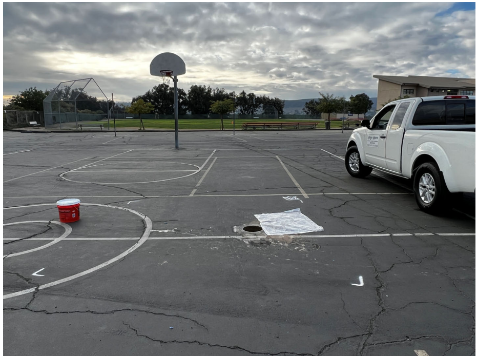
Photograph 2: View of East Hardcourt play area looking south. Note the several AC cracks running in the north-south and east-west orientations.
