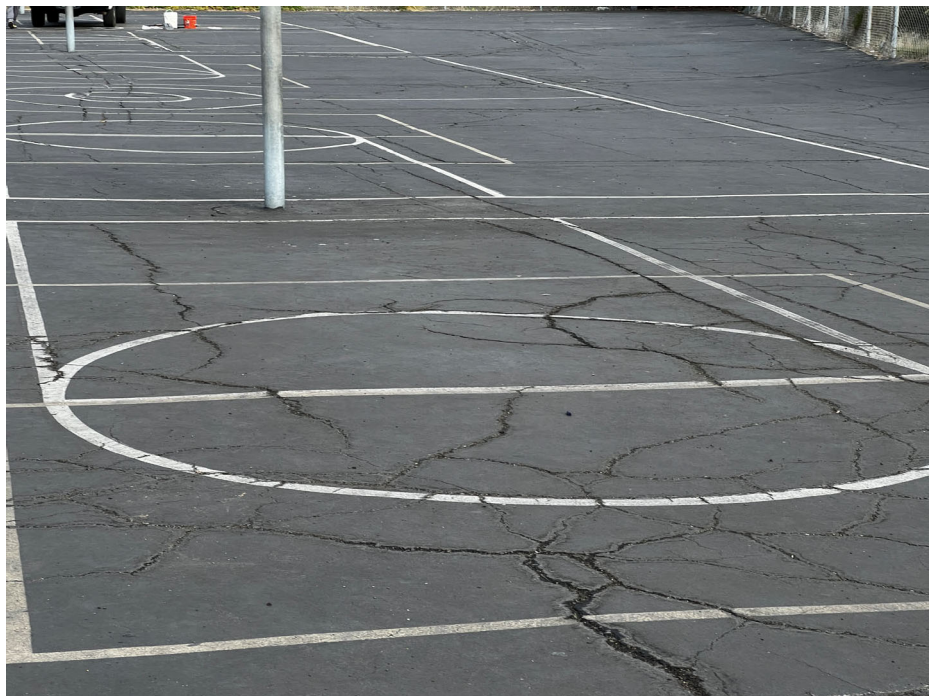
Photograph 4: View of several random oriented cracks in the AC with various cracks that have previously been patched and have reopened.
